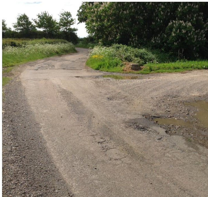
Consistent lack of care has led to some unsafe sections of road – I have asked for urgent repairs for basic safety.
